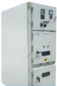
VCB (Vacuum Circuit Breaker)
