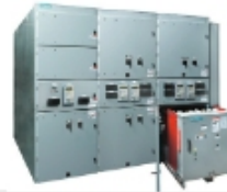
Medium Voltage VCB Panels (MV Switchgears)
